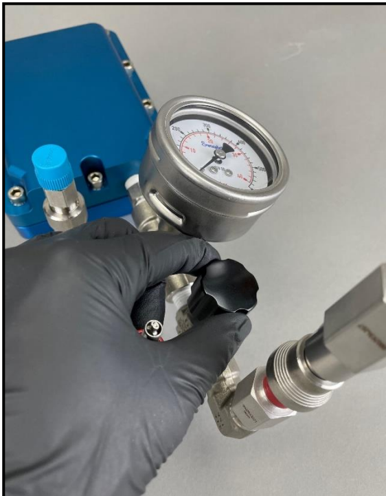
Figure 11. Inlet Valve opened.
